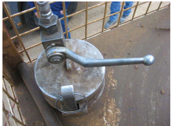
3" Cam lock fitting used to inject compressed air into refuelling pod
