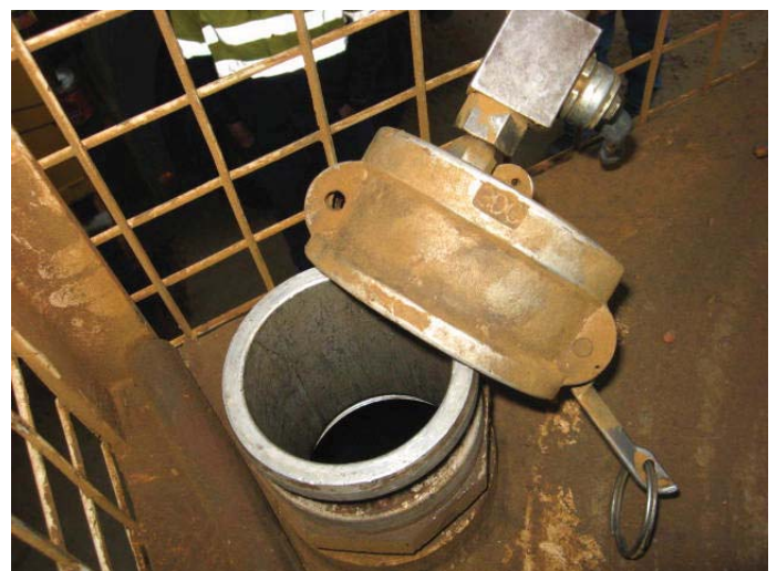
Close up of 3" Cam lock fitting used to inject compressed air into refuelling pod
