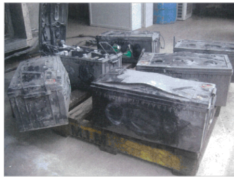
Batteries from the ERB
