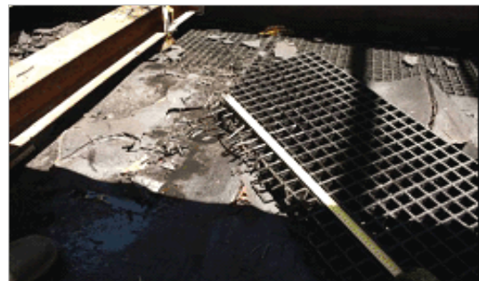
Condition of the fibreglass grid mesh
