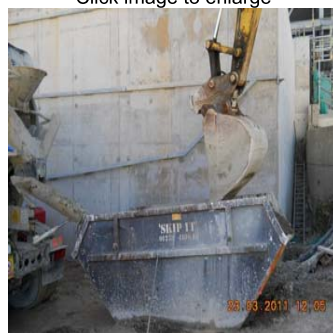
Poor Delivery Set Up
