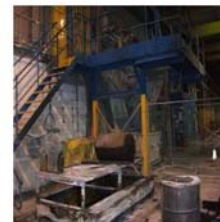
oil storage bund
