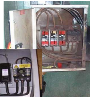
Panel after short circuit
