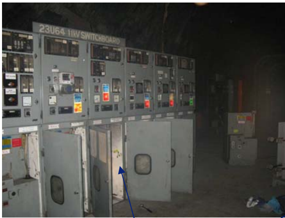
Panel 5, Shutter damage from arc flash
