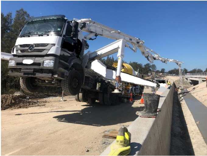
Photo 1 - Uncontrolled movement of concrete boom truck
