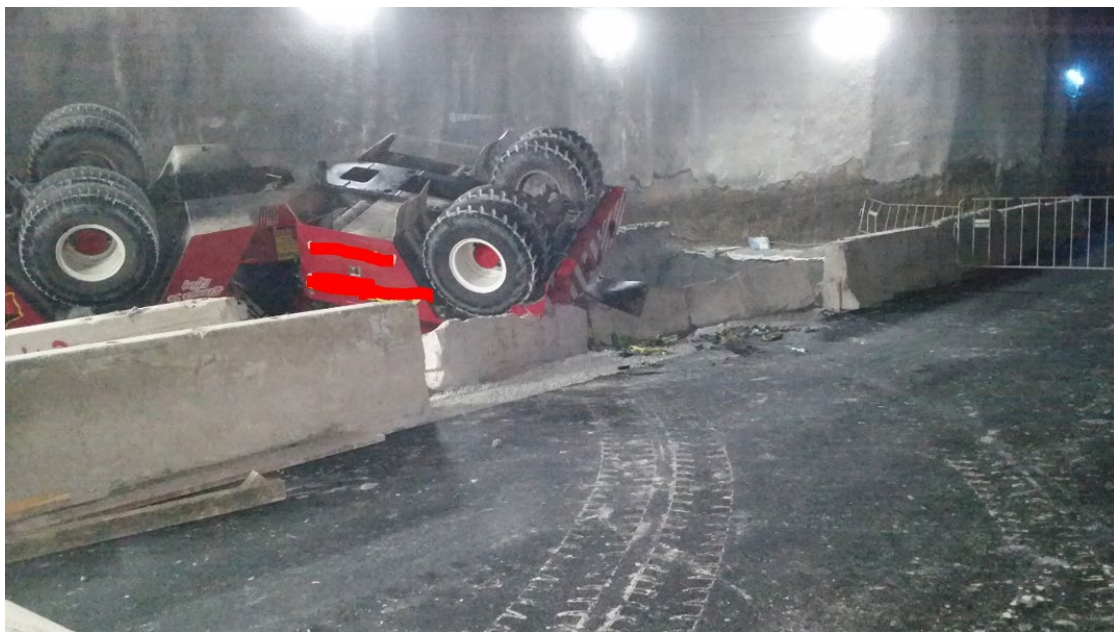
Photo: 25t Terex articulated mobile crane rolled over onto the roof and edge of the shaft. Tyre mud marks on the asphalt indicate the crane location prior to incident.
