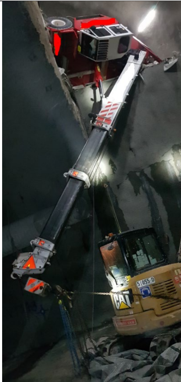
Photo: From the base of the 10m deep shaft, looking up to the 25t Terex articulated mobile crane
