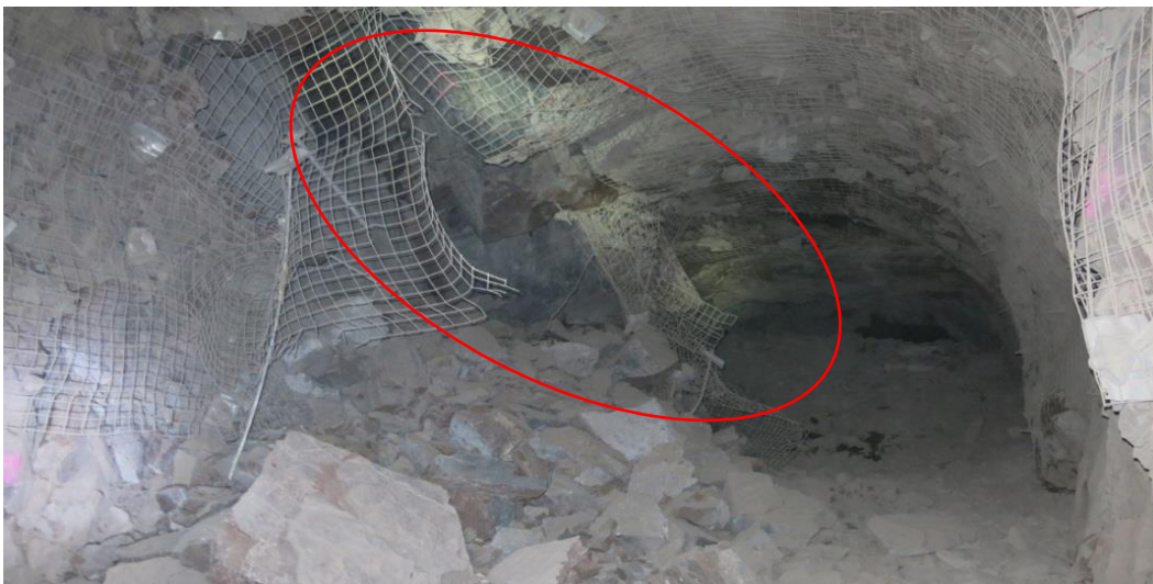
Figure 1: Strainburst from the left shoulder and resulting rockfall.
