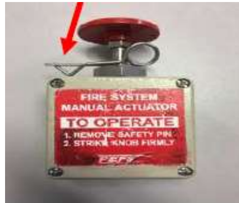
Pin leg crossed over and cannot be removed
