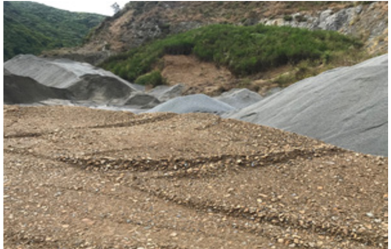
Photo: No berm on the tipping edge
