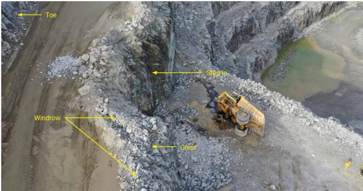
Narrowing section of roadway. Note the deviation in the pit wall profile resulting in a 'step in' on the wall reducing the running width of the ramp.
