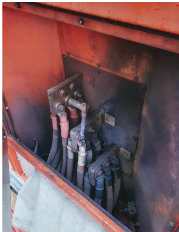
Portable load bank involved in the incident
